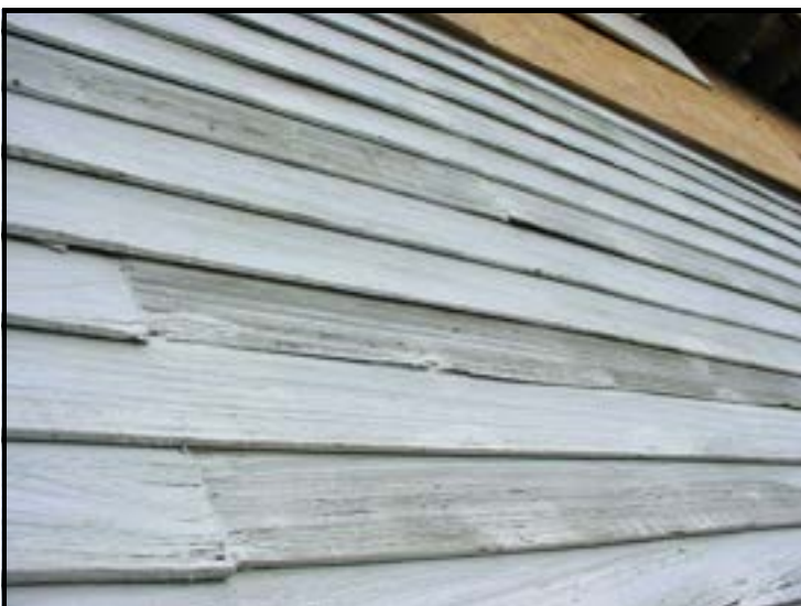
This photo shows a close-up of the siding on the west wall above the servery and ell porch. The damage done by power washing can be seen here where the wood was washed away, leaving some boards very thin. In extreme cases, it is possible for power washing to wash a hole through the wood.
