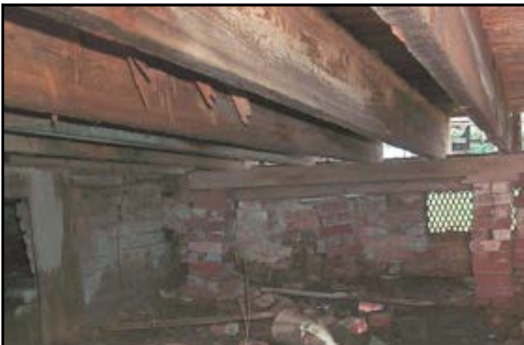
The photo at left shows the exterior foundation wall from underneath the house before restoration began. Prolonged water exposure had caused the mortar to deteriorate and the foundation wall to collapse. Brick piers had been built to support the house framing. This photo was taken from the Historic Structures Report for Lakeport Plantation.
