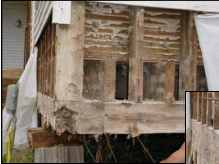
The photo at left shows a deteriorated sill beam at the southwest corner of the main house. In the close-up below, the deterioration has left a corner post tenon exposed.
