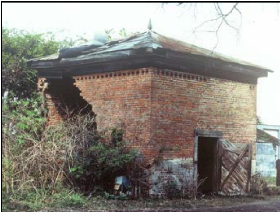
The original Lakeport smokehouse, seen in the photo at left, fell sometime during the 1980's. When this photo was taken, the west wall had already begun to collapse. This photo was provided by descendants of the Johnson family.
