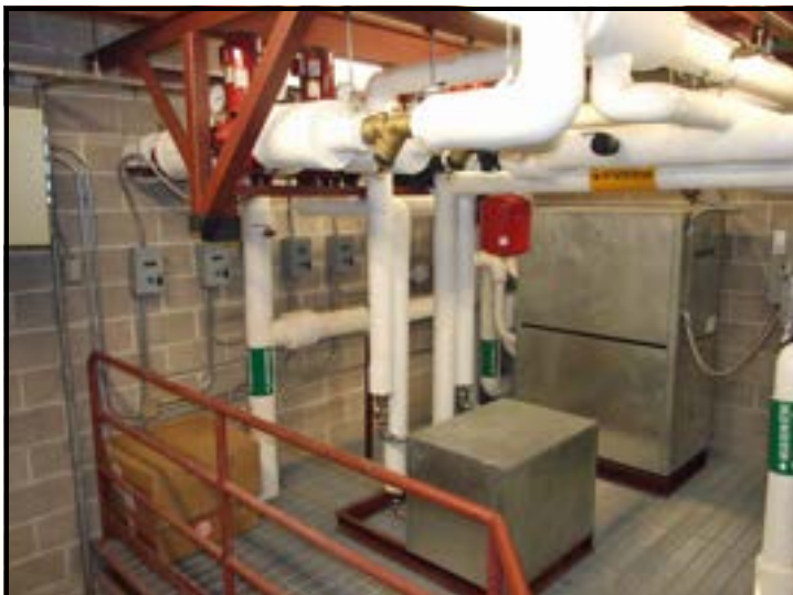
The photo at left shows the hydronic piping and pumps which direct the feed from the geothermal field to the mechanicals inside the smokehouse.
