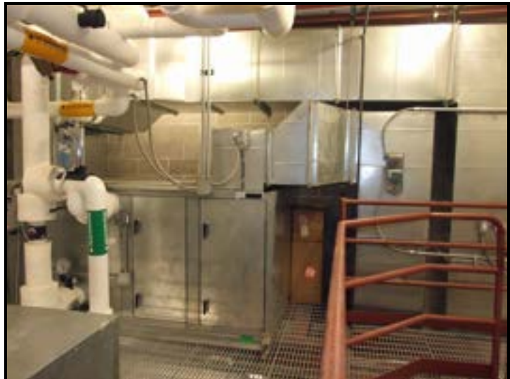
The large air handler can be seen in the photo at right setting on the mezzanine floor of the smokehouse. The supply and return air ductwork comes from the floor below to tie into the air handler.
