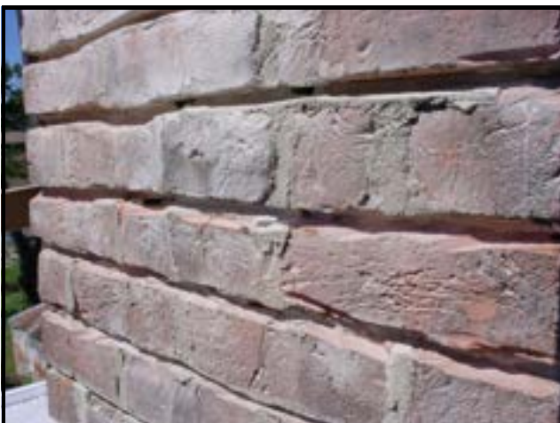
This photo shows the damage that was done to the historic bricks when the mortar was removed with power tools rather than hand tools. Damaged bricks had to be removed and replaced.
